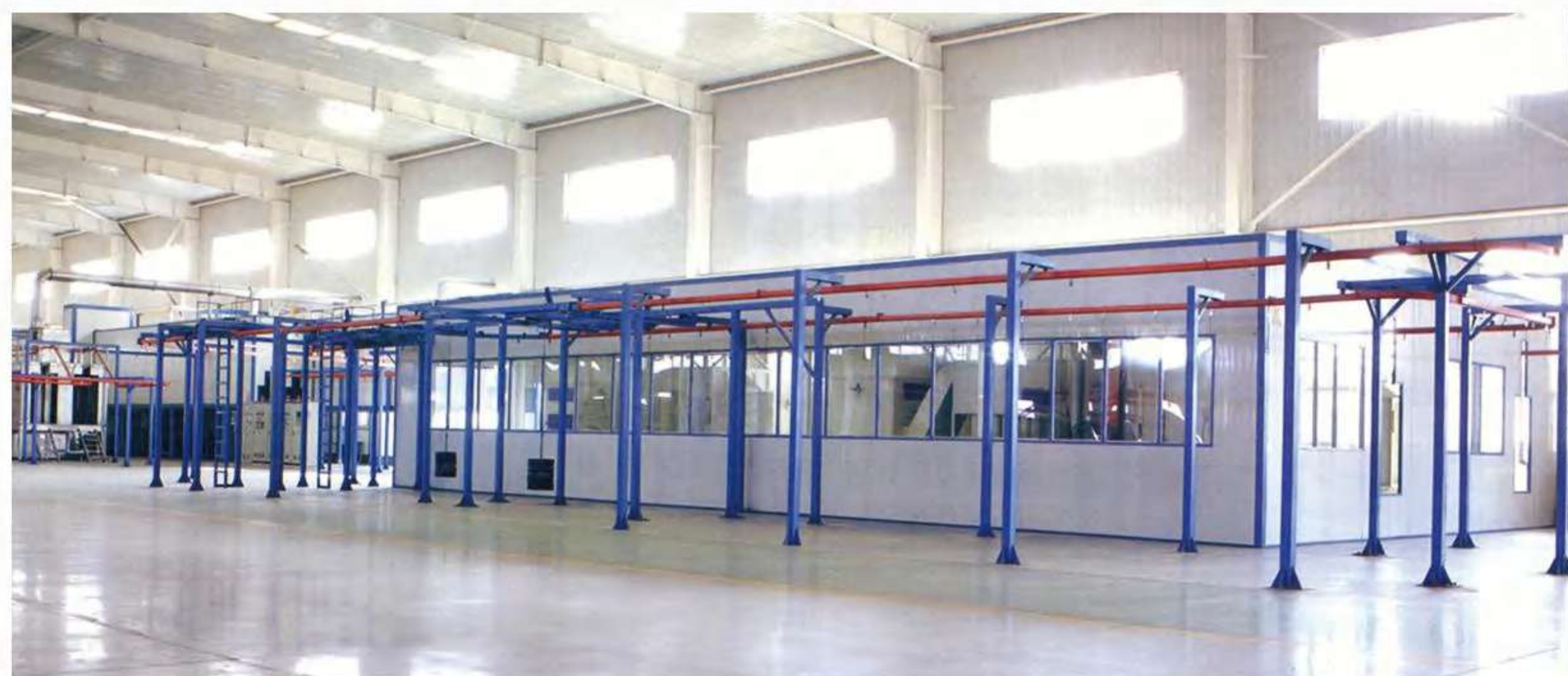
喷涂流水线 Spraying line
